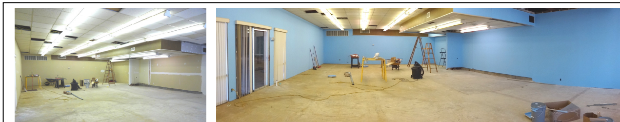
Here is a dramatic example of some significant progress in preparing the new ASMR train layout facility on Westwood for occupancy. On the left is the room as it appeared, unpainted, after removal of some unwanted structural elements and taping and bedding the sheetrock. On the right is the room after painting by Ken Riediger, Jim Gibson and Tony McKinney during the afternoons of May 24/25. The open ceiling panels are where Kent Stark, Cecil Walston, Scott Fritz, Ben Diamond and Chris Bisset have been installing new wiring.
